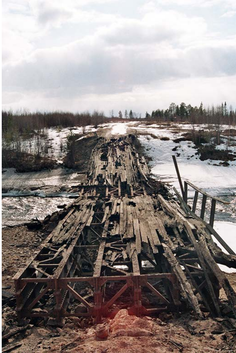
Illustration 16: Bridge burned down by poachers on the gravel road between Verchnetulomsk and Kovdor. Poachers protect themselves from hunting inspectors by the systematic breaking of roads (oral information from hunting inspector Zajkov, April, 2003) (photo: Lukas Allemann, 2003).
